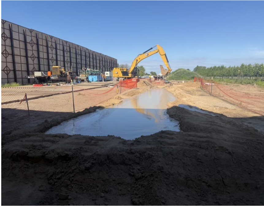
Facing west near MP 3.0, receiving full returns to the exit pit on HDD P4-5
