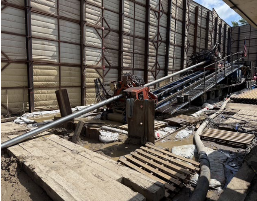
Facing north near MP 2.4, completing the 30-inch-diameter ream pass on HDD P4-5
