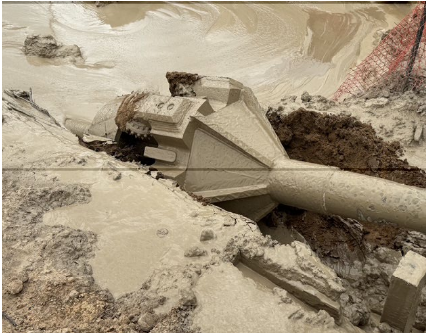
Facing south near MP 3.0, commencing the 42-inch-diameter ream pass on HDD P4-5
